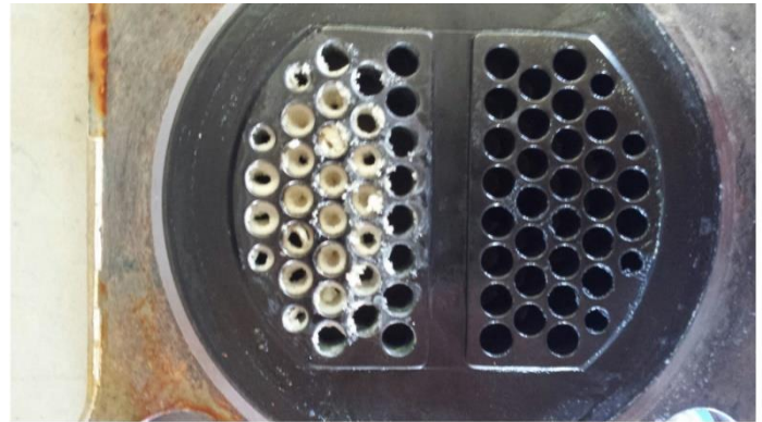
Figure 13 - Pipeline flow meter plate with clogged orifices due to precipitated plaque
