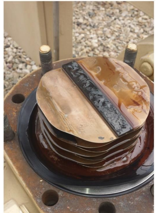
Figure 10 - Gas meter plate, saturated with oil
