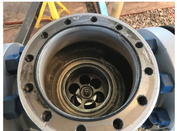
Figure 11 - Pipeline gas meter
