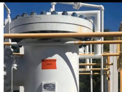
FIGURE 12 Processing plant inlet filter.
