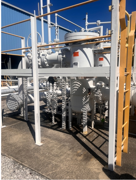
Figure 13 Processing Plant Inlet Filters
