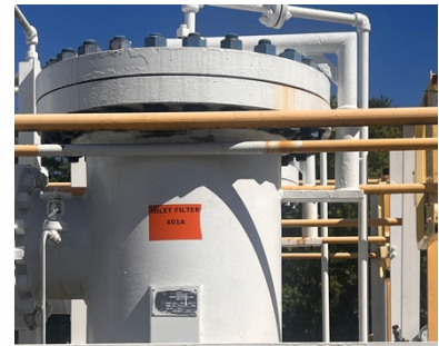
Figure 12 Processing Plant Inlet Filter
