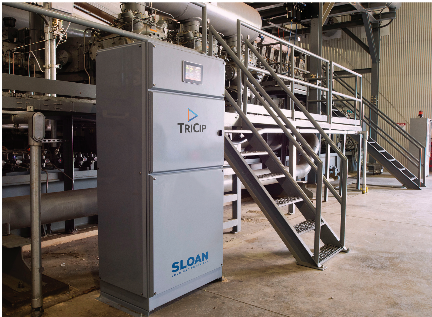
The TriCip Lubrication System Installed On A Separable Compressor
